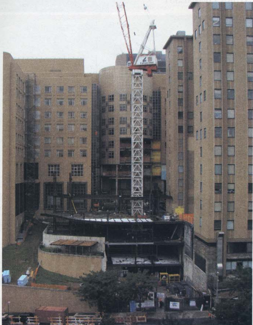
Work on the 120,000-sq-ft facility includes two phases of new construction and one phase of renovations to existing structures.
