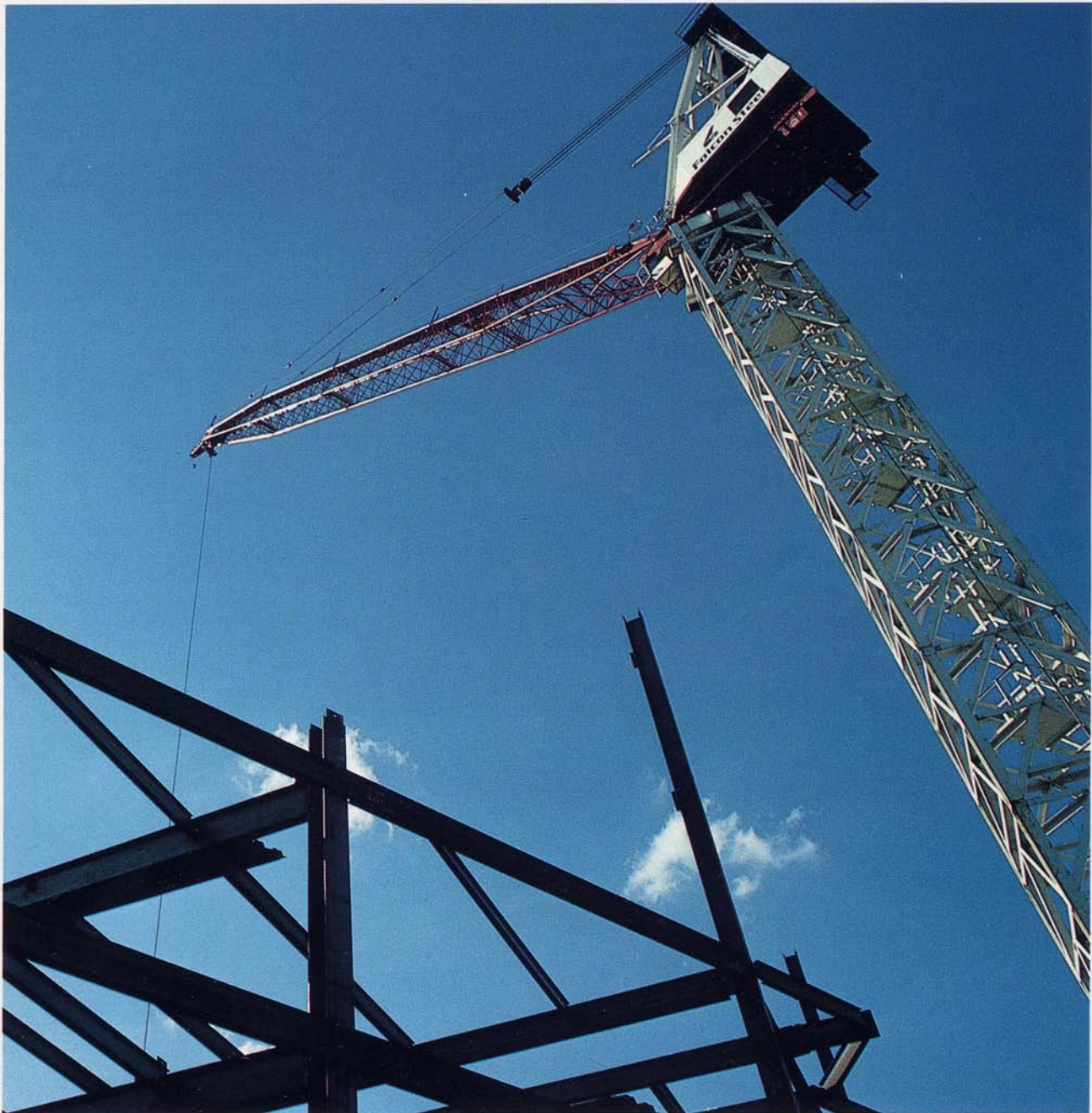
12-story superstructure steel and 3 levels of steel below grade were erected quickly through careful planning and crane equipment selection
